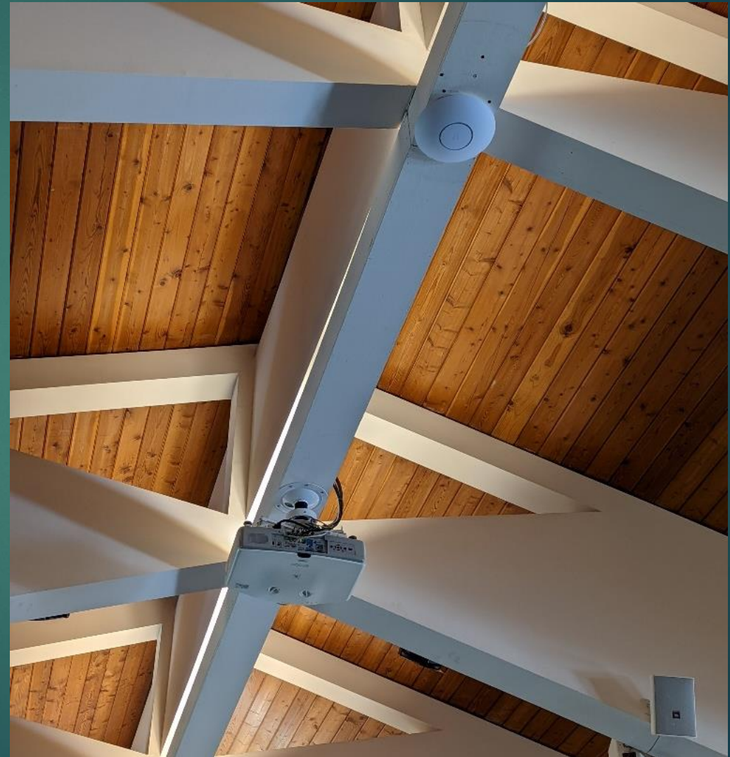
Above: Meeting Room new Wi-Fi access point
